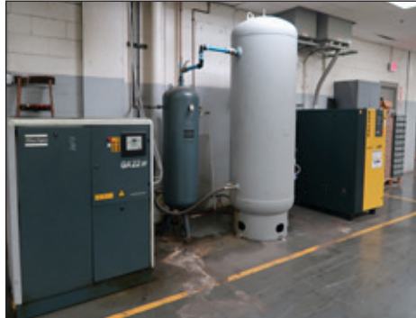
ATLAS COPCO GA22FF & KAESER AS30T AIR COMPRESSOR
