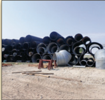
INVENTORY OF CAUSEWAY PIPE
