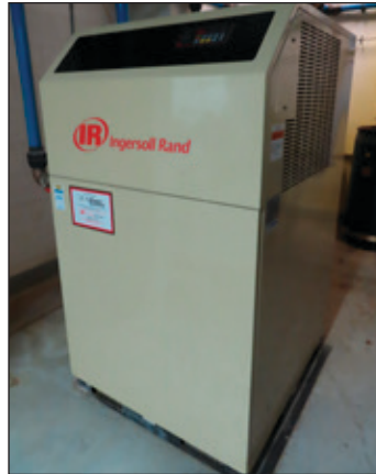
INGERSOLL RAND COMPRESSED AIR DRYER
