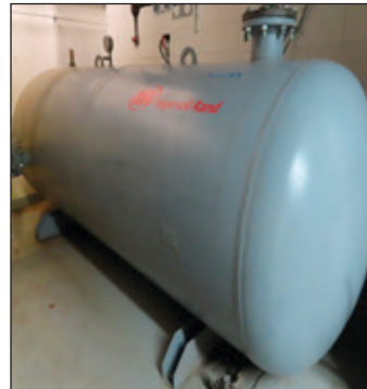
INGERSOLL RAND AIR RECEIVER TANK
