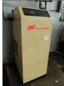
INGERSOLL RAND COMPRESSED AIR DRYER
